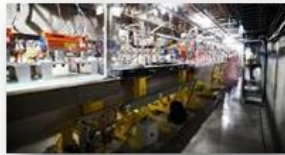
FACET Beam Test Facility
